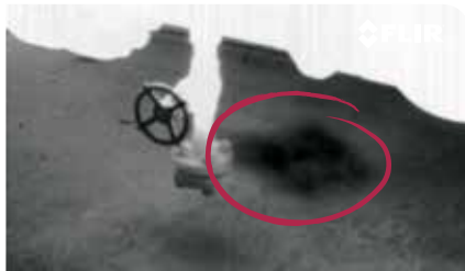
Captured gas leak from production site.
