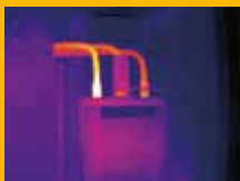
Poor connection and internal damage
