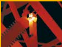
Incorrectly secured connection
