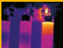
Internal fuse damage
