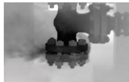
Figure 2: OGI allows users to spot the source of leaks, such as in this valve.
