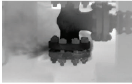
Figure 4: Image of Leak from a Valve
