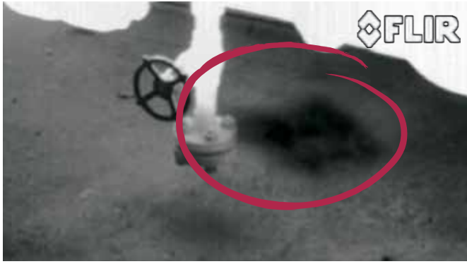
Captured gas leak from production site.
