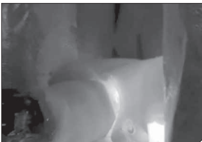
Leak in a 4-way valve dryer skid
