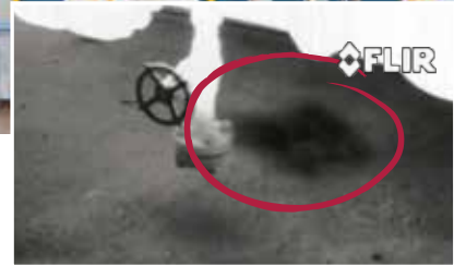
Captured gas leak from production site.
