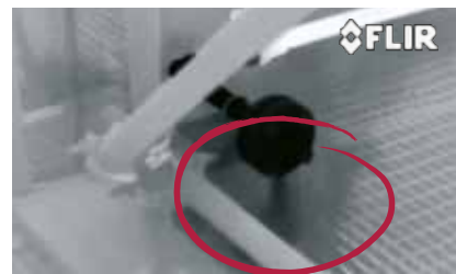
Gas leak is clearly visible on the thermal image.
